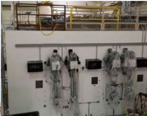
Newly refurbished hot cells for alpha-processing
