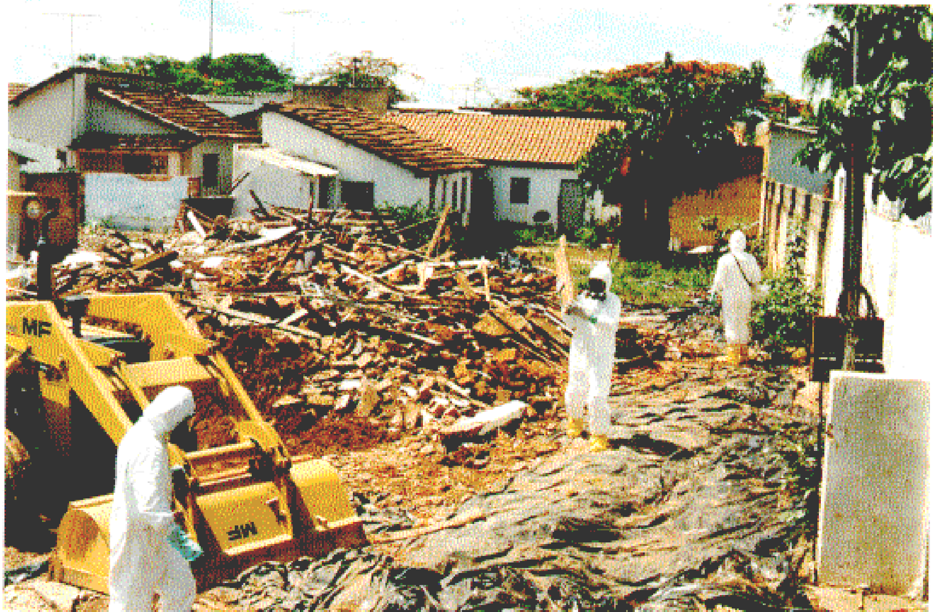
Contaminated rubble from a house
