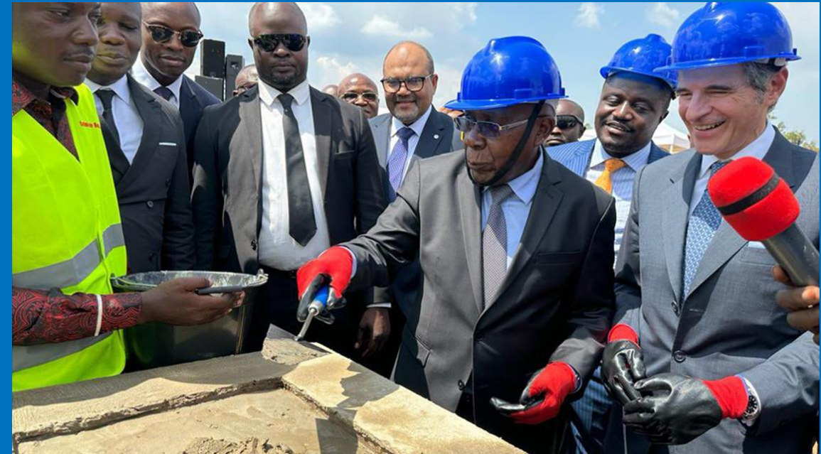
Laying the foundation stone of what will be the first public radiotherapy centre in the Democratic Republic of the Congo, November 2023
